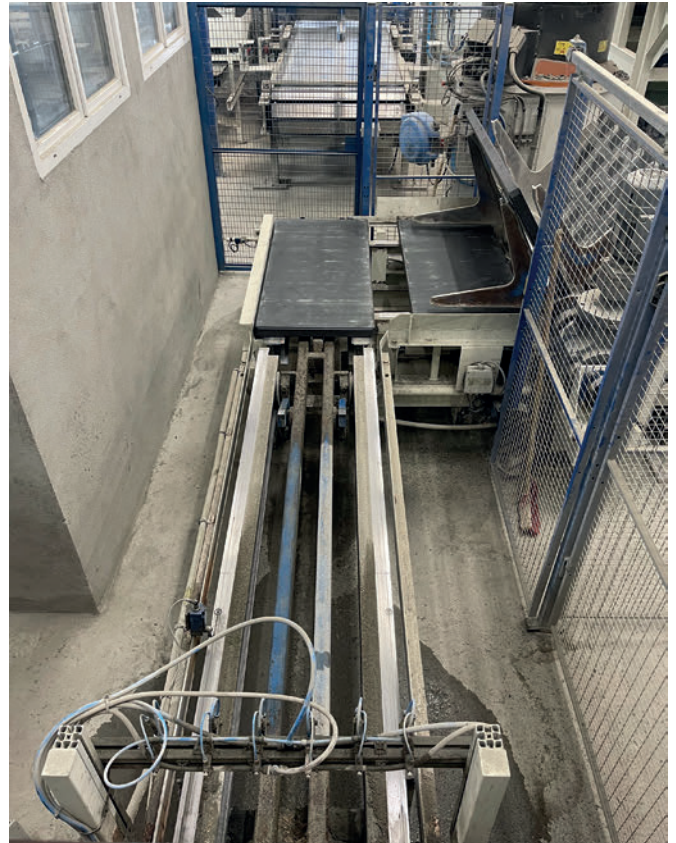
Quadra Q6 circulation system with Wasa Uniplast Ultra today
